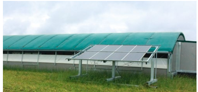
Power supply of a mobile chicken shed
