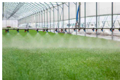
Agricultural greenhouse water supply system
